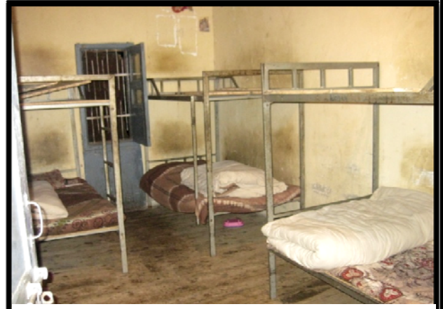
The dull rooms with discoloured walls
